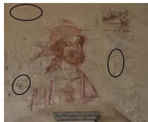
Fig. 5.Picture showing small cracks and holes in the wall
